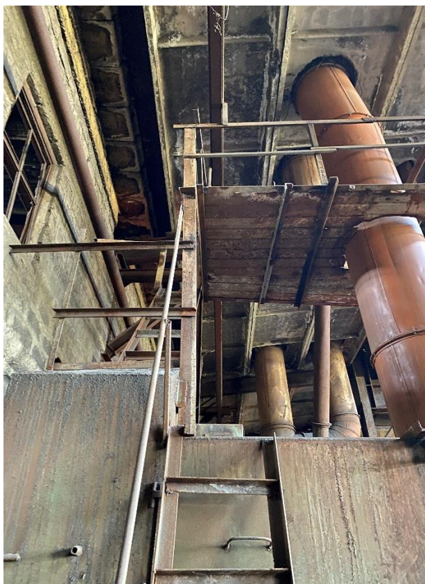
Stack left side with measuring platform
